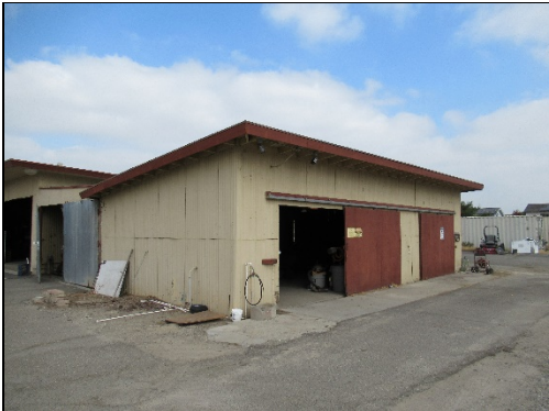
Equipment Storage Shed, south (left) and east (right) elevations, view northwest (LSA 2021)
