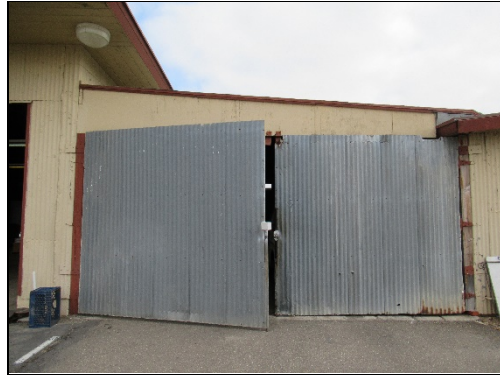
Shed between Maintenance Shop and Equipment Shed, south elevation, center projection, view north (LSA 2021)
