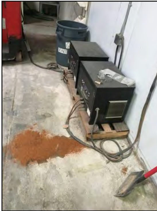
Electric forklift battery charging station in the Hybrid Apparel warehouse
