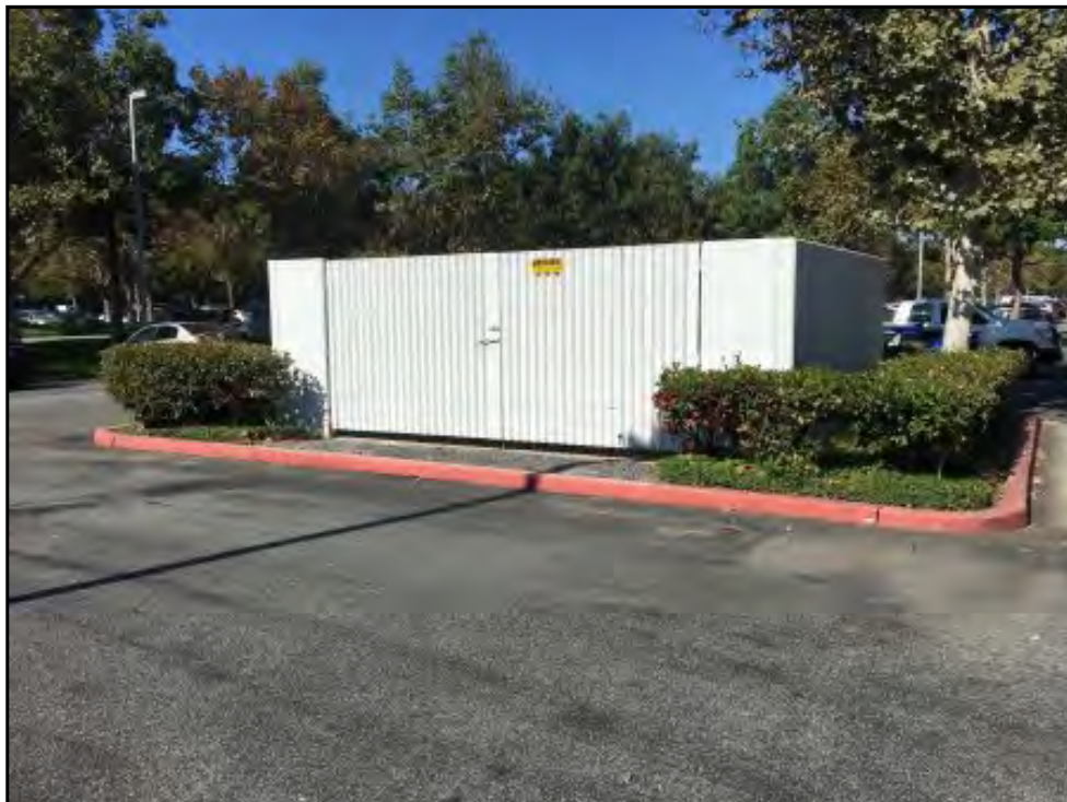
Electrical transformer, SoCal Edison
