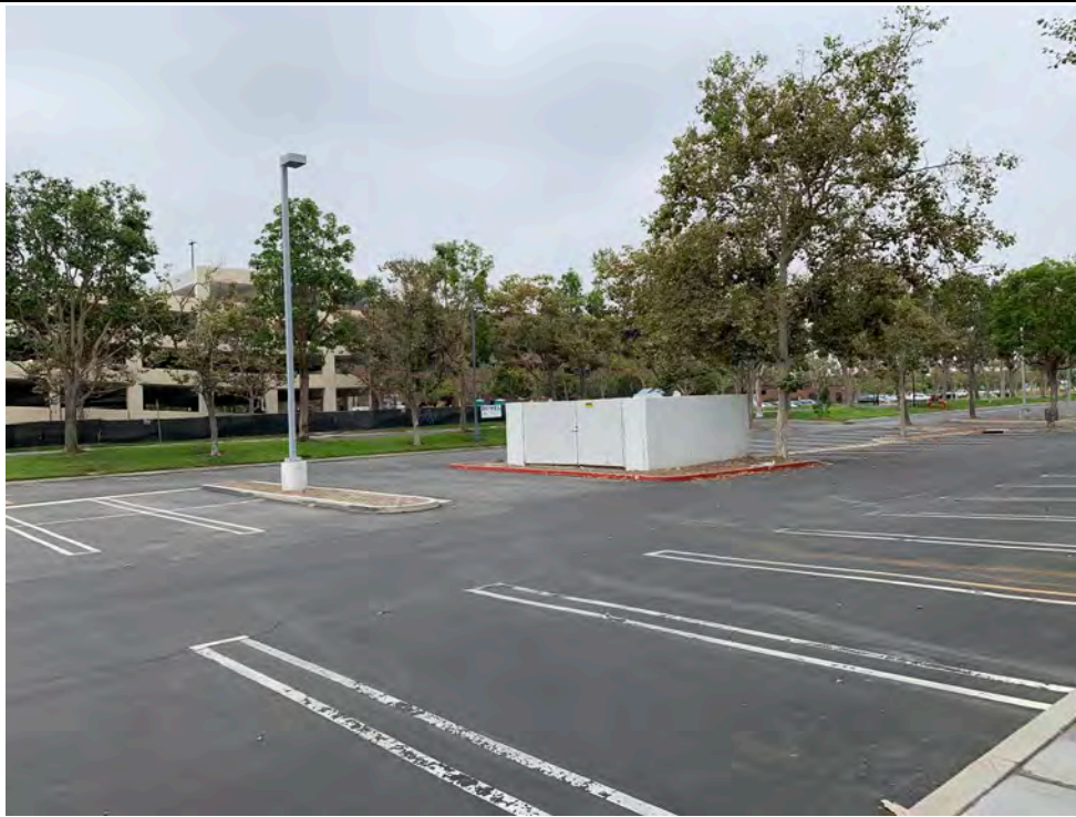
Photo #7 View of the locked transformer enclosure located in the southern parking lot of the 5757 Plaza Drive building.
