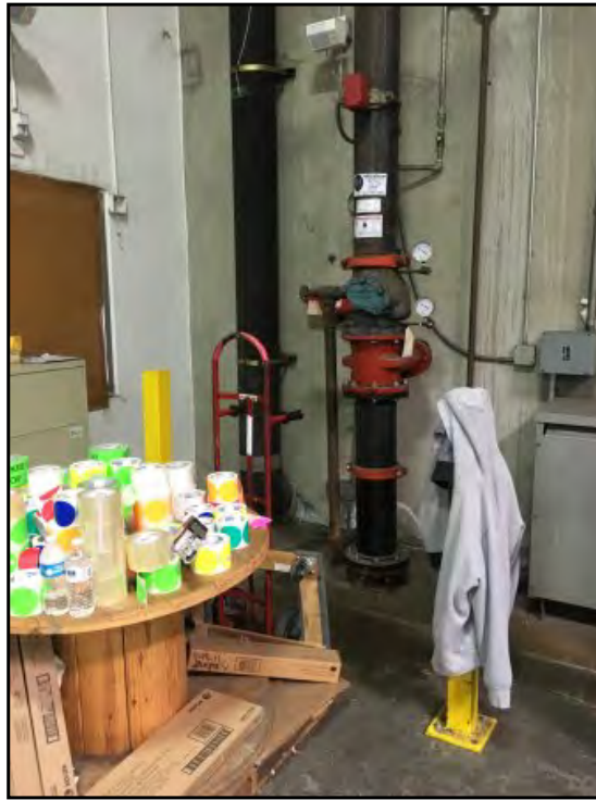
Hybrid Apparel warehouse fire suppression supply
