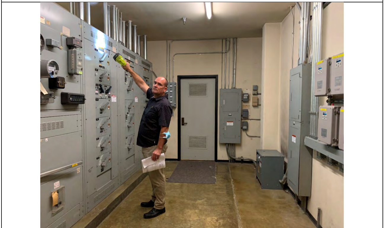
Photo #6 View of the electrical room of the 5757 Plaza Drive building.
