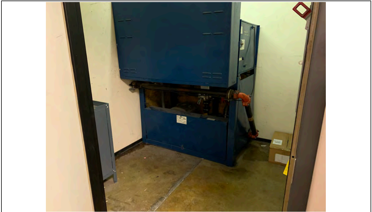
Photo #5 View of the elevator maintenance room of the 5757 Plaza Drive building.
