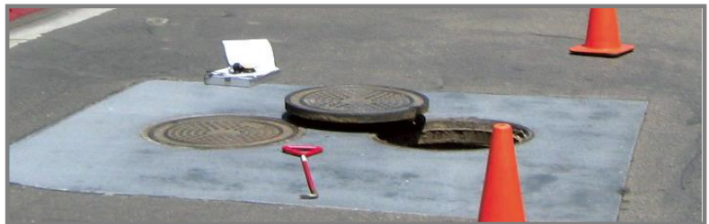
Units typically accessed through 2 or more adjacent manholes
