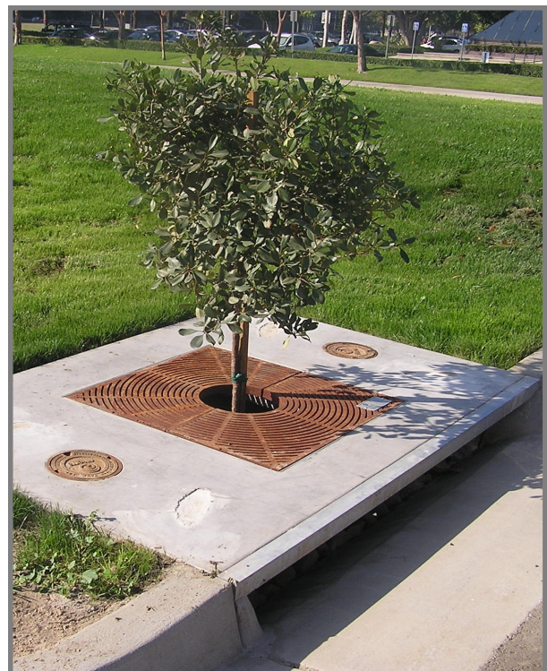
Filtrerra Bioretention System
